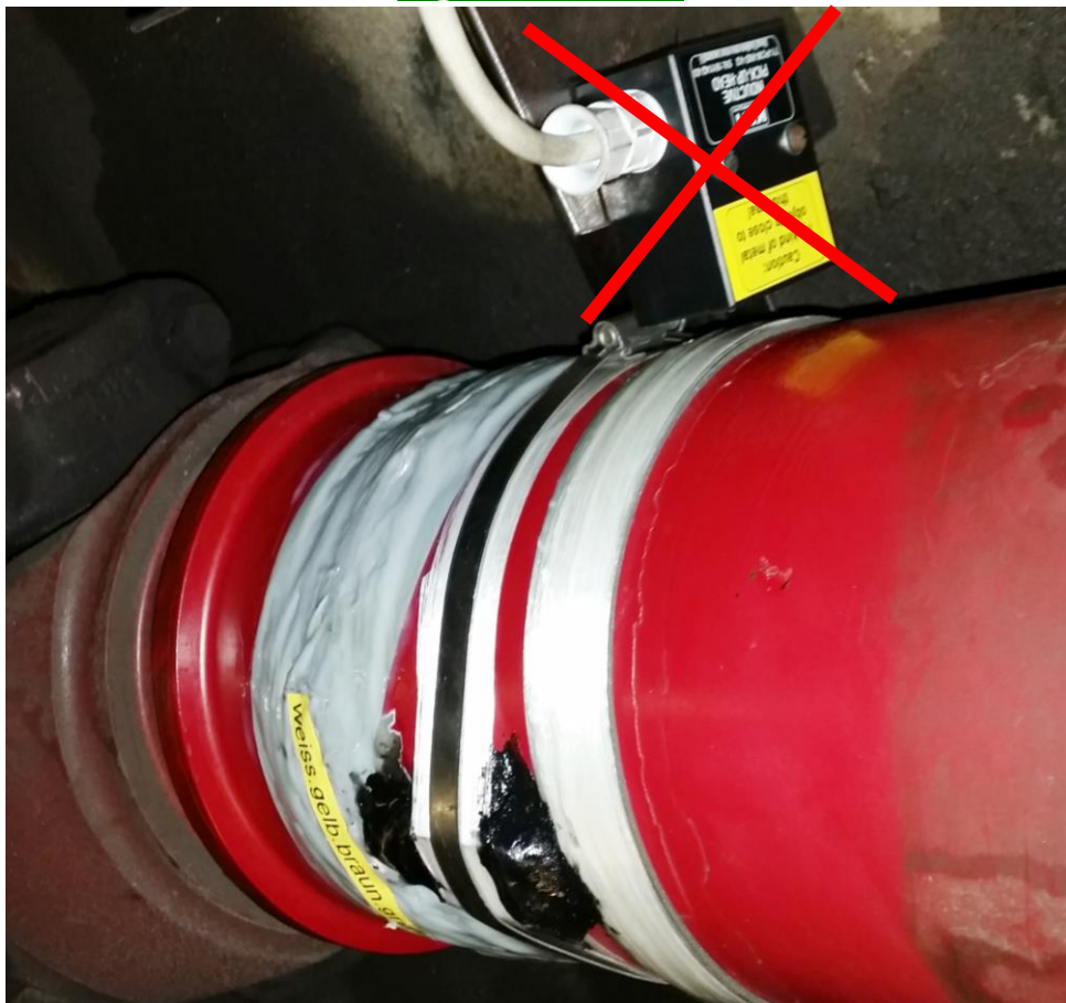
Wrong installation, head position is 90° wrong to the coil and will not work!
